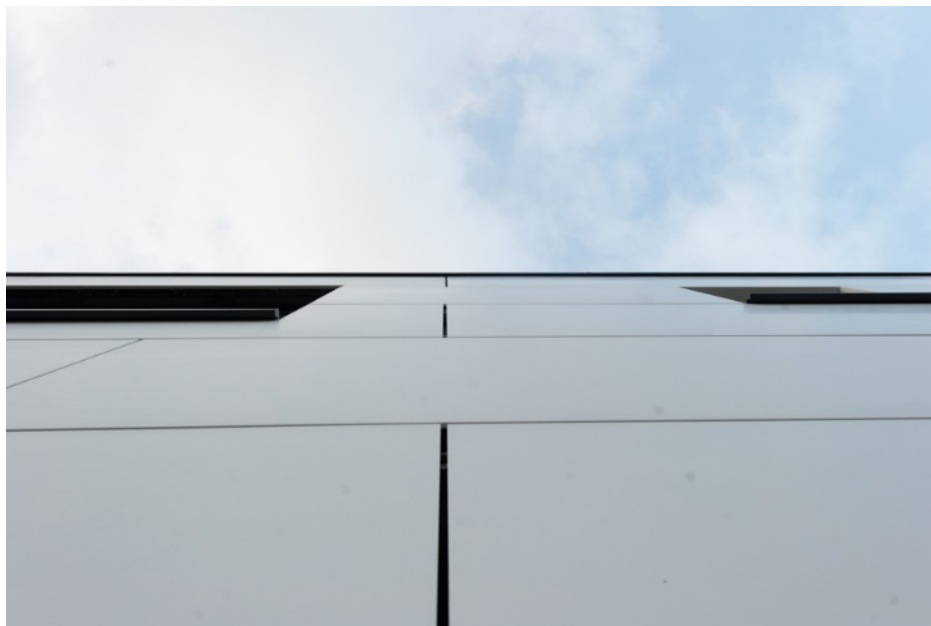
The fine, black seams of the facade made of DuPont™ Corian® yield an equally modern and timeless look for the “Glazialhaus” in Hamburg, Photo: www.behringstrasse126.de , all rights reserved.
